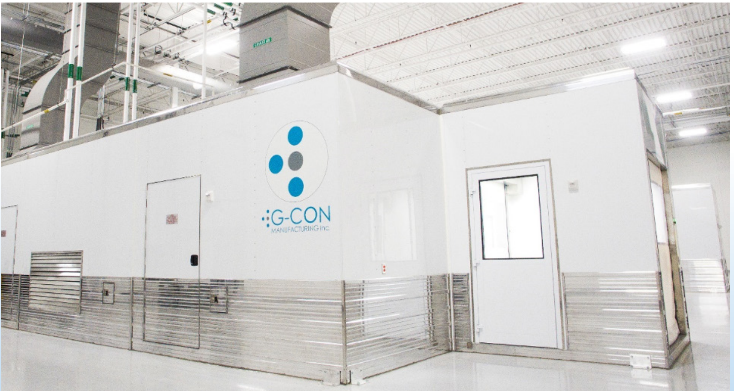
The outside of an assembled modular cleanroom facility, built within an existing industrial building. Note the HVAC, plumbing and electrical interconnections between the cleanroom modules and the enclosing building.
